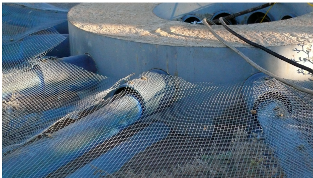
Figure 1: An example of PVC radials that have fallen from their desired position.
