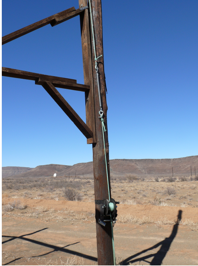
Figure 11. A similar picture from the site showing the spring in series with the line approach. Note the length of the tails on the double overhand knots.
